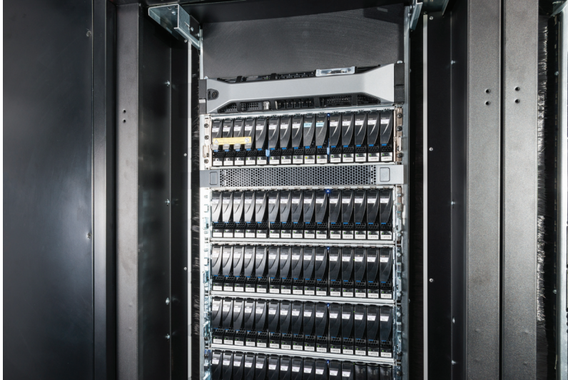
Figure 11.14 A storage array.
